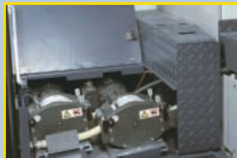
Installed on the UV varnish tower coater of MAN Roland R700 series printing presses, twin baseplate-mounted 701 pumps have reduced downtime and increased production speed. One pump accurately meters the water-based varnish from a container to a weir on the press, the other scavenges excess varnish for re-circulation.
