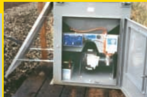
UK railroads experience problems every fall when trackside trees shed their leaves. This installation uses a Watson-Marlow Bredel pump to feed gel-borne sand to the rails and increase grip for the trains
